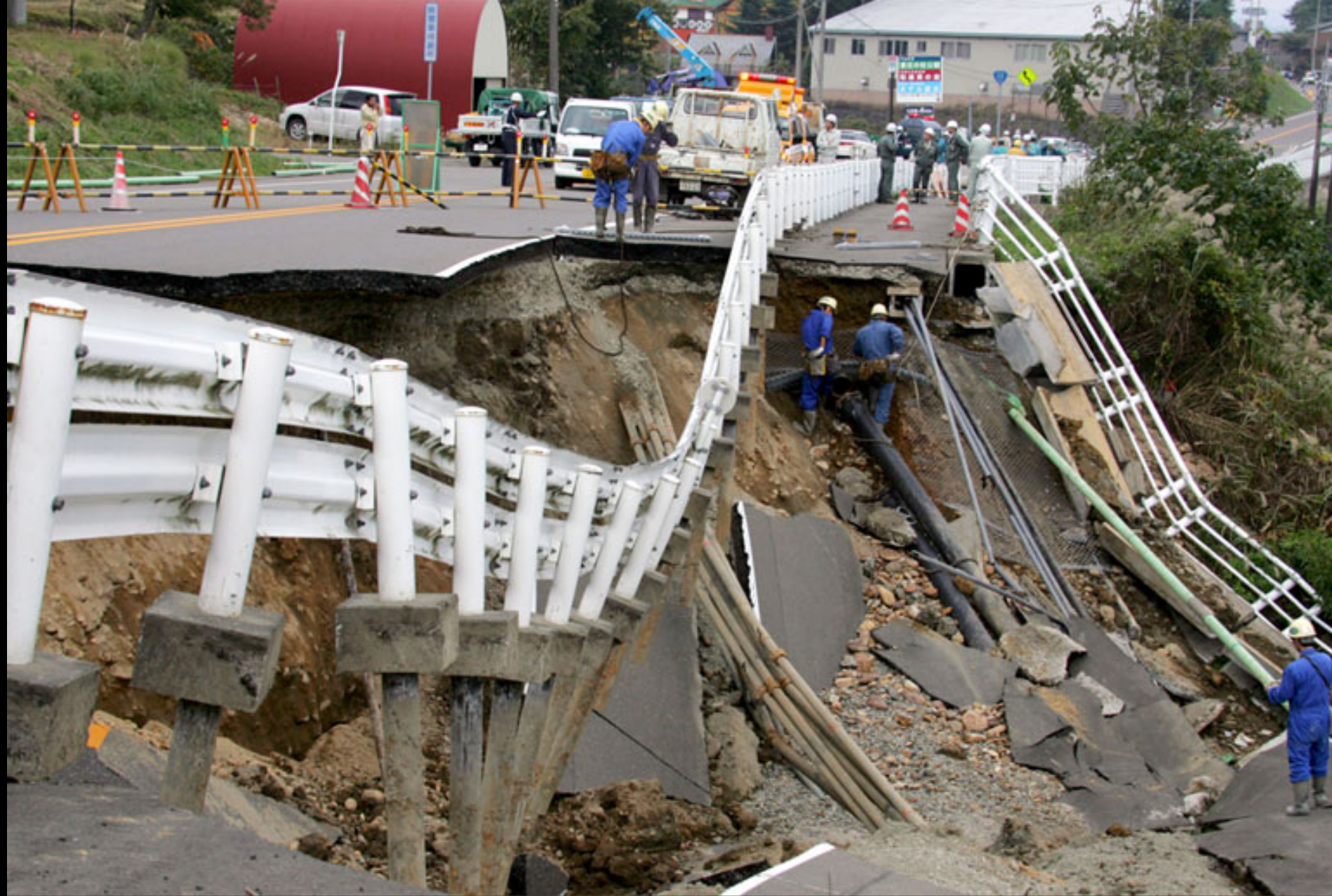
Aftermath of an earthquake in Japan, 2004 Photograph by Kimimasa Mayama/Reuters
